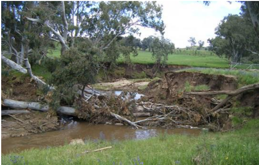
Some of the damage along the creekline at 'Jilliby' following the 2010 floods (photo courtesy of Rob Kuiper, Riverina Local Land Services)
