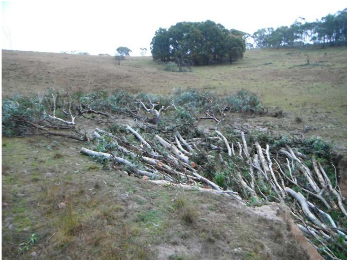
Figure F3: Heavier logs, wire and stakes help to weigh down and hold the surface brush-matress in place. Logs staked on contour just below the face and a careful final packing are critical. A 'tangle' of branches above the face will protect both grass growth from grazing and the cuttings of poplar which have been planted in an offset pattern.
