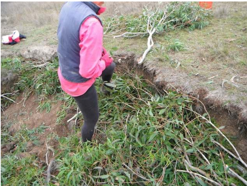
Figure F2: Brush is carefully packed against the face and under the lip of the A horizon. This helps to intercept any undercutting flows and provides reinforcement if and when soil does break off. This process should be repeated on any damage in the future.
