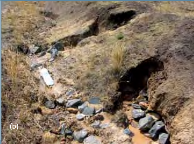
Figure 26. Undercutting and collapse of roadside batter due to construction of a table drain in dispersive clay. Note the failure of the blue rock rap to prevent further erosion.
