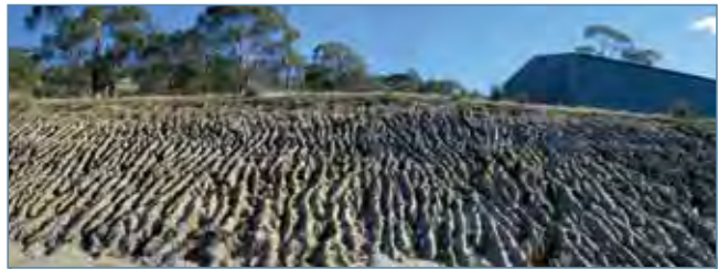
Figure 17. Extensive 'outlet initiated' tunnel and rill erosion caused by excavating a cut and fill pad for a large building in a dispersive soil. Triassic sandstone parent material.
