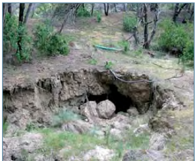
Figure 34. Piping failure of a dam constructed from soils derived from Permian mudstone, Penna area. This dam is known to have failed on first filling. The image was taken from the dam floor, looking at the inside of the dam wall.
