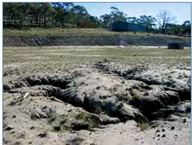
Figure 18. (Same site as Figure 17) Tunnel erosion in footings intended for a large building. Erosion resulted from ponding of rainwater on highly dispersive fill. The fill contains a number of narrow slots (up to 1.2 meters deep) caused by surface water 'dissolving' through the footing.
