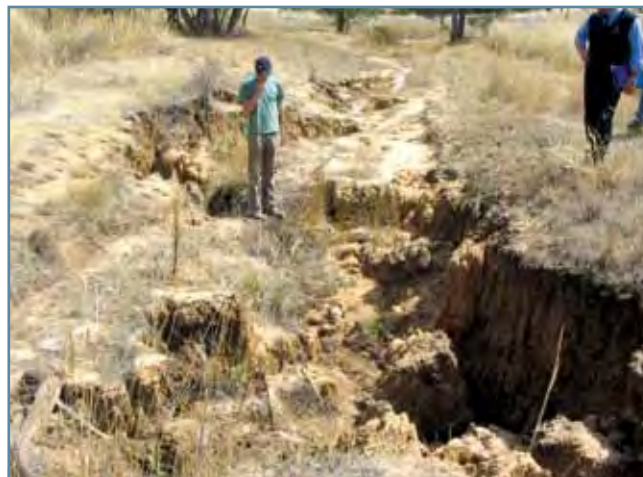
Figure 24. Tunnel erosion resulting from construction of a stormwater culvert in dispersive clay derived from Triassic sandstone, Brighton.
