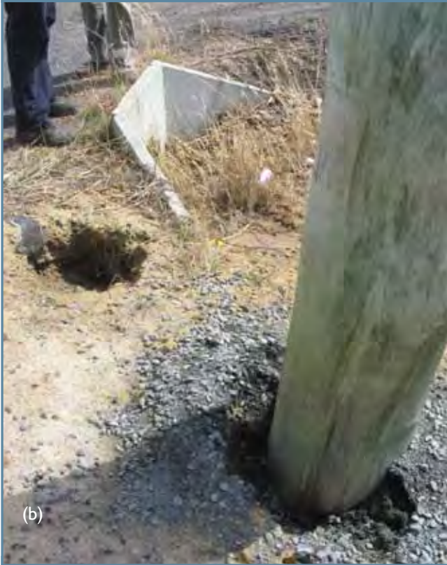
Figure 21 (a) Tunnel erosion initiated by installation of an optical fibre cable into a dispersive soil. (b) Subsidence and early stages of tunnelling resulting from inappropriate installation of power pole in a backfilled trench.
