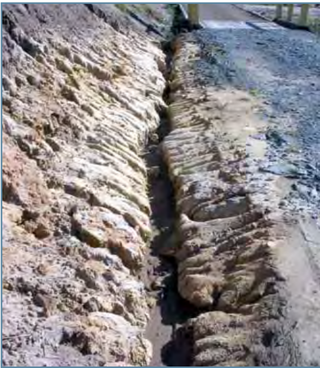
Figure 27. Table drain constructed in dispersive subsoil. The concentration of runoff in the culvert is greatly adding to the erosion problem, resulting in slumping and undercutting of the road and the adjacent batter slope. This photo was taken 18 months after the driveway was constructed.
