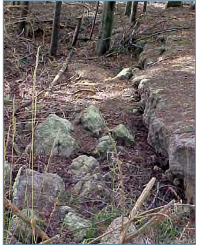
Figure 8. Collapse of tunnel roof, following loss of dispersive soil horizon leading to formation of a stable depression, Cygnet.
