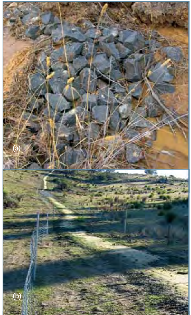
Figure 36. Examples of tunnel erosion control (a) Poor technique. Rock rap is usually an inappropriate erosion control technique for dispersive soils. Normally rock barriers work well to trap sediment and reduce erosion. However in dispersive soils, hard surfaces such as rock are quickly bypassed i.e. upper corner of the rock structure (b) Excellent technique. Note the entire repaired area is fenced, and the whole length of the repaired tunnel is covered with topsoil and jute cloth. Sand barriers have been constructed every 20 meters down the slope.
