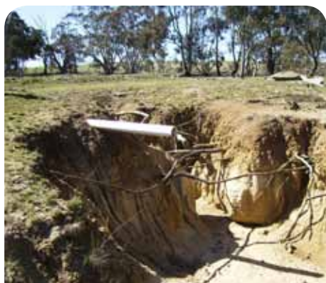
Figure 4.5: This State 2 woodland was already susceptible to erosion, but incorrect placement of this runoff diversion pipe (middle) probably made it much worse. The pipe was allowed to discharge water at a height, displacing large amounts of soil.
