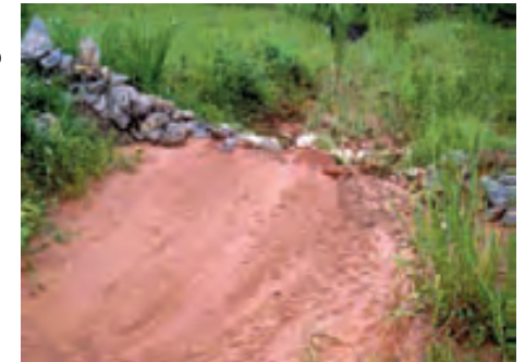
Sediment needs to be removed to maintain the effectiveness of this structure. Source: Michael Frankcombe IECA
