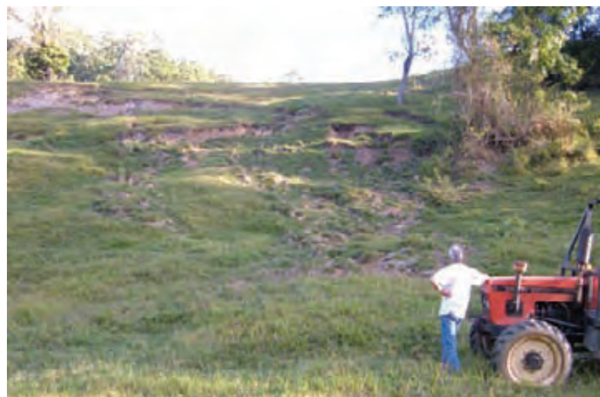
A deep-seated slump on a wet slope
