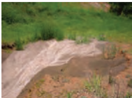
A sediment fan means erosion upslope.
