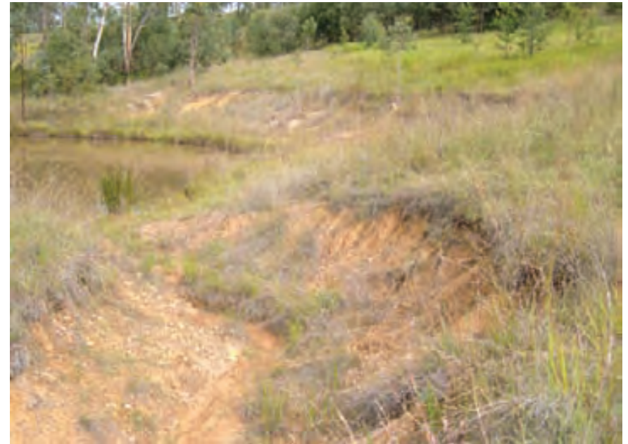
This eroding spillway needs repair.
