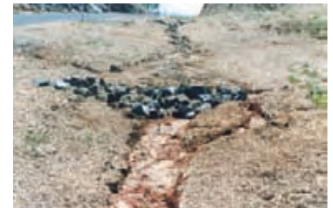
This rock check dam is failing because the rock does not extend far enough up the channel sides, and the lowest point is not in the centre.
