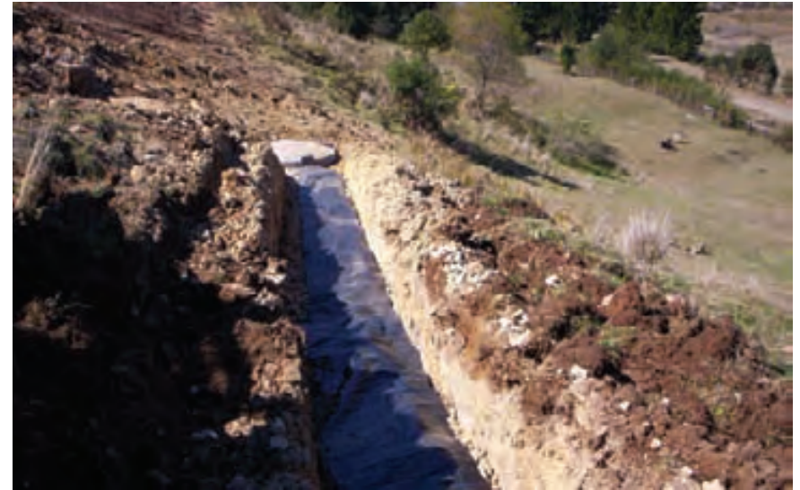
A large subsurface drain upslope of a landslide collects water for disposal elsewhere.
