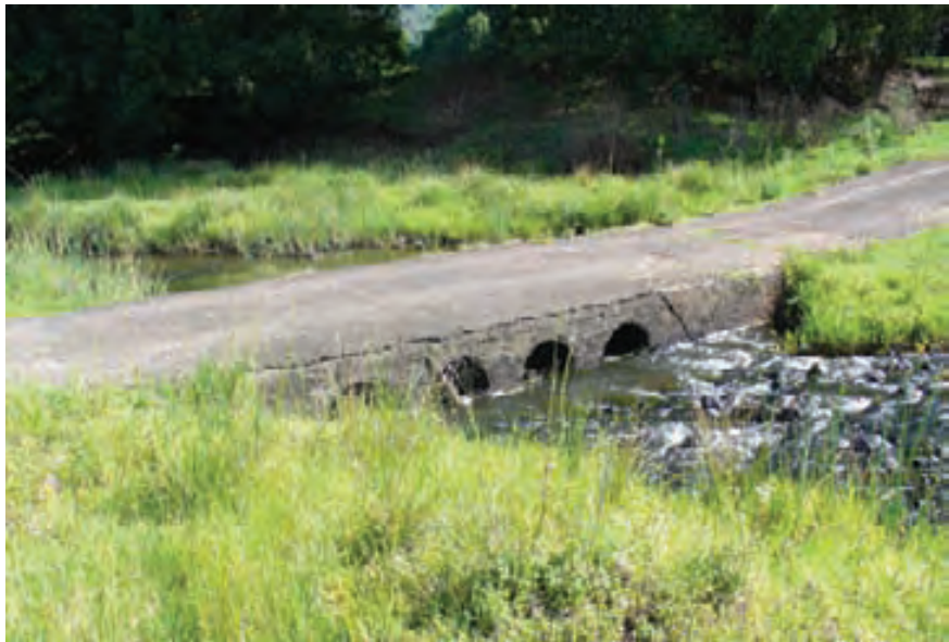
This older style culvert crossing is designed to function as a causeway in high flows.
