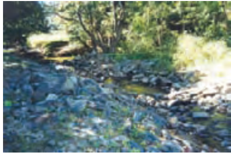
A rock check dam Source: Michael Frankcombe IECA
