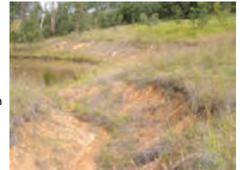
An eroding dam spillway
