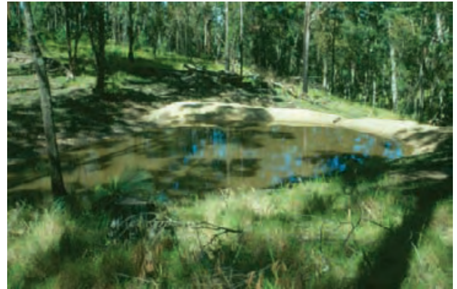
This embankment has overtopped because of insufficient freeboard between the embankment crest and the spillway (to left). Source: Mark Stanton-Cook NSW DPI
