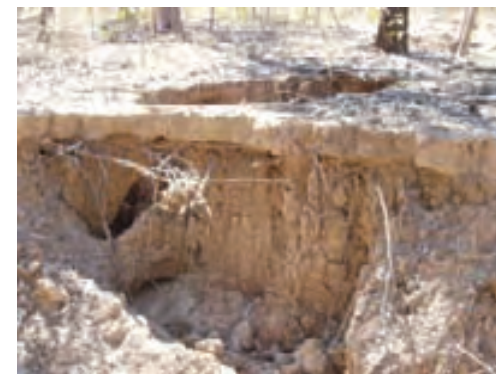
Tunnel erosion Source: David Morand DECC
