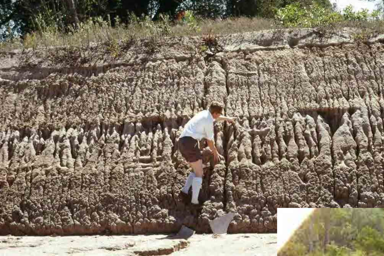
Erosion on batters of road cuttings with dispersive soils
