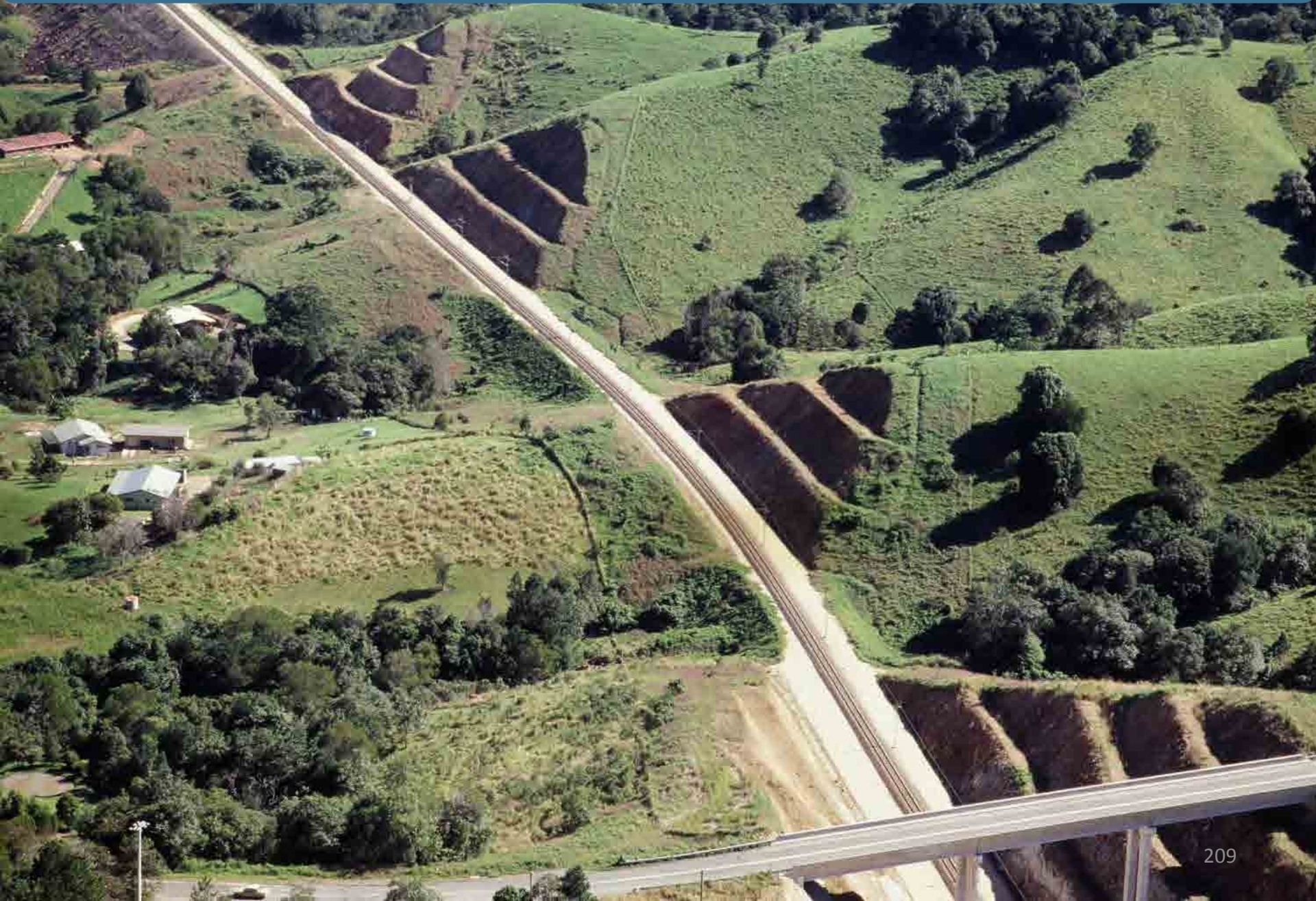
Batters are formed when rail or road cuttings are required to create level surfaces in hilly land.
