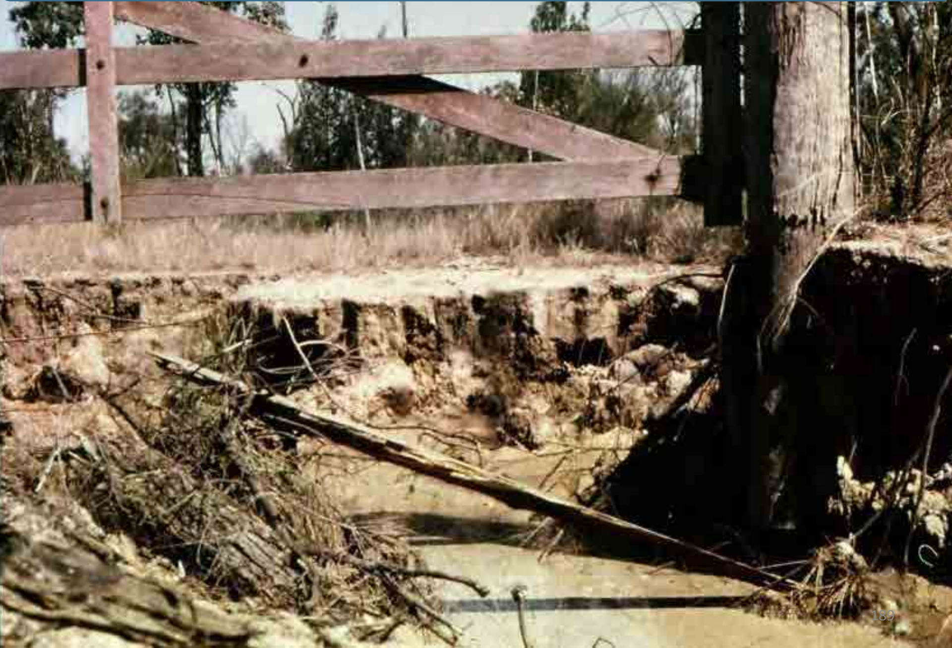
Erosion causing severe damage to a road at a gate entry in dispersive soils south of Bogantungan, central Queensland (note the prismatic structure in the exposed subsoil)
