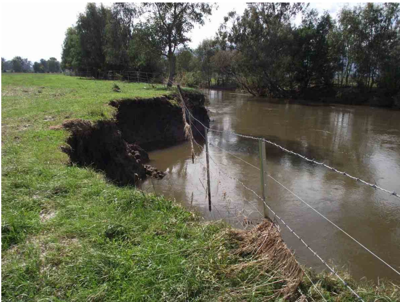
Figure 5.1 – What can happen to a riparian fence when it's located too close to the channel, Jeremal Creek (north-east Victoria) after the 2012 flood (photo: North East CMA)
