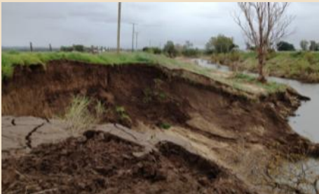
Mass failure, or slumping, occurs when chunks of the bank slide or fall into the stream, often leaving near vertical banks.
