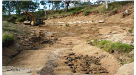
Stabilising the toe and retaining existing mature vegetation on the bank as well regenerating vegetation in the early stages of establishment (foreground) can form part of your plan.
